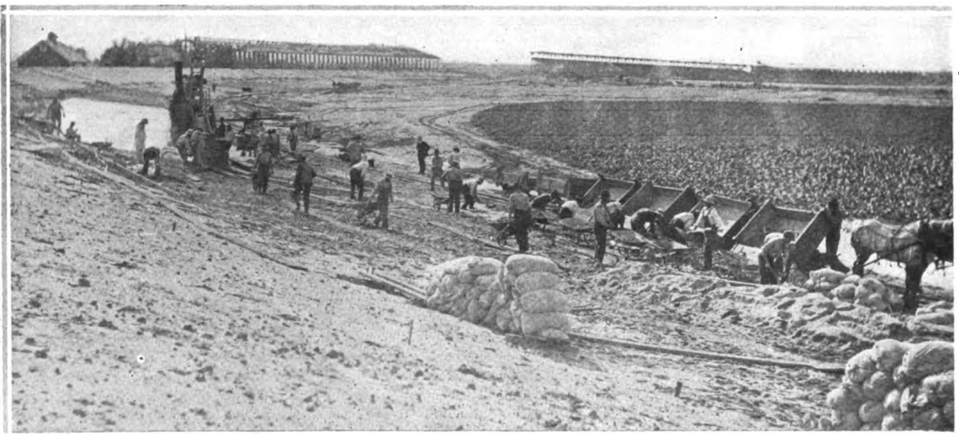
Building the Twin City Motor Speedway. The illustration shows how the work of excavation and the grading and surfacing of the track are being carried on at the same time to facilitate the completion of the course. Note the grandstands under construction and nearly completed in the background. This course is near Minneapolis and St. Paul, Minn.
